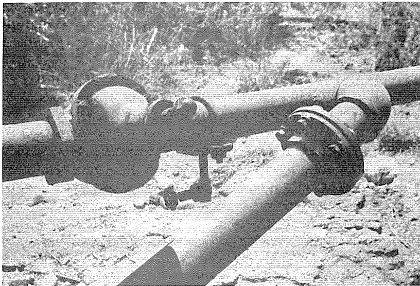
FIGURE 10 A LOOK AT THE PIPE FITTINGS NEAR STORAGE TANKS.
